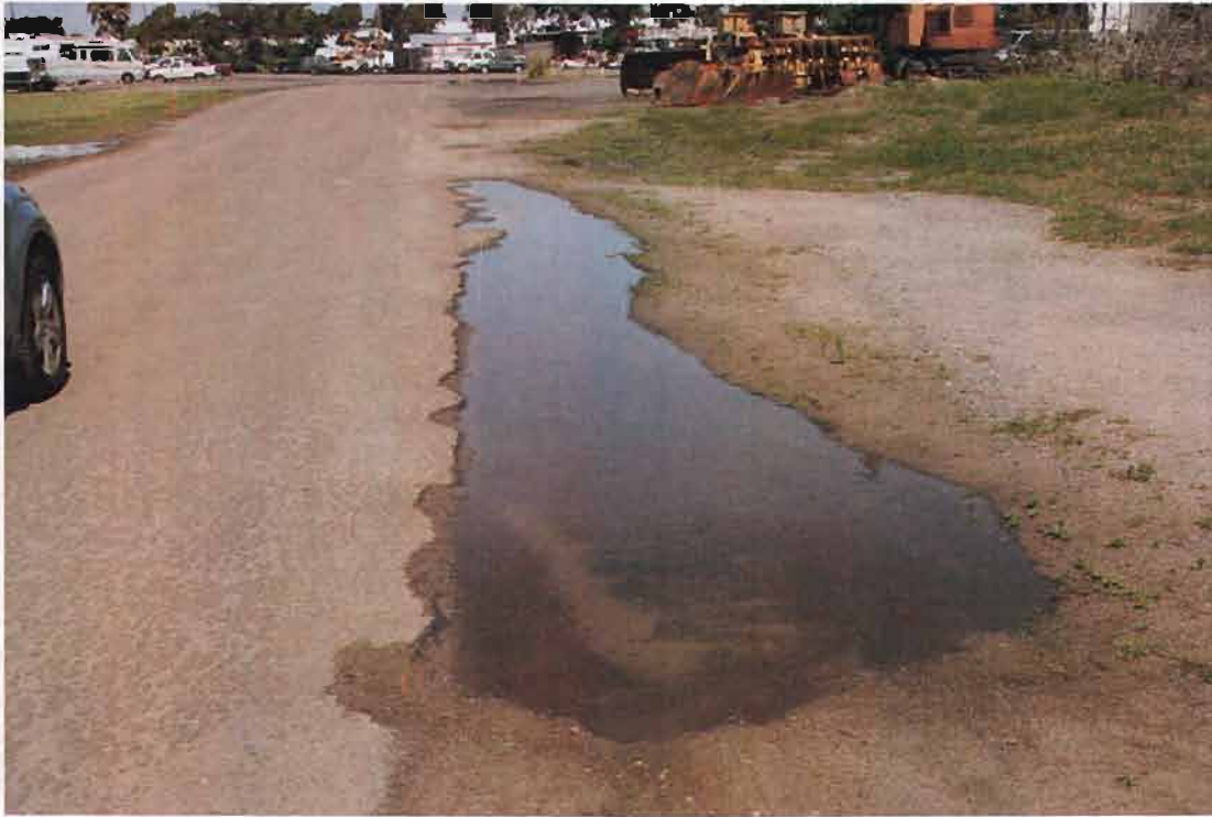
PHOTOGRAPH 15: View of Feature Q looking north showing shallow ponding within roadside depression.
