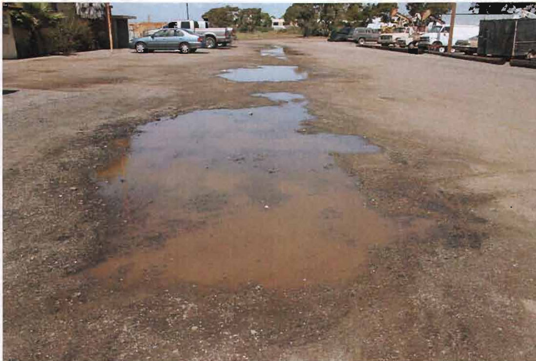
PHOTOGRAPH 18: View of Feature U looking north showing shallow ponding in asphalt parking area.
